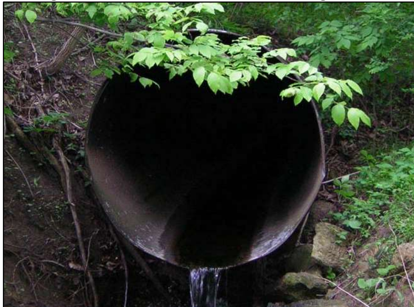
Figure 11: MS4 outfall location with illicit discharge
