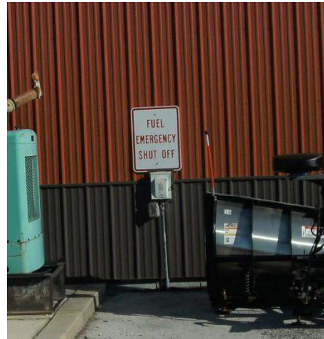
Figure 3-7. AST emergency shut off
