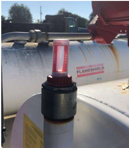
Figure 3-6. AST leak detection system at fueling station
